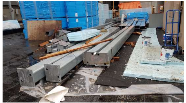
A common sight on any project - uncovered membranes used as a staging area.
