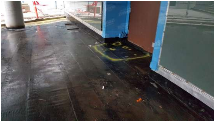
Many small penetrations were found around doorways, the damages were caused by primer dripping onto the membrane
