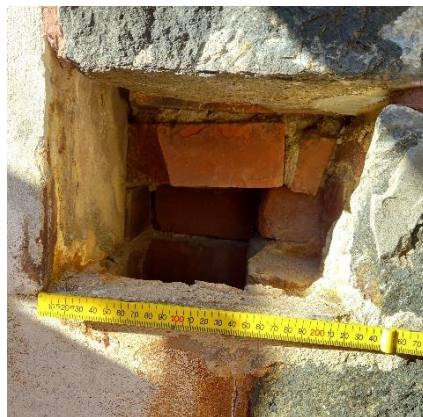
Image 5: Exterior masonry exploratory opening revealing double wythe brick back-up wall. (WSP Applied Sciences Building, University of Otago, NZ, 2021).
