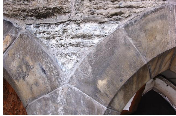
Image 4: Evidence of efflorescence at window stone surround
