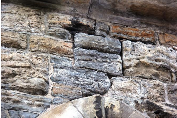
Image 3: Mortar deterioration and loss below decorative banding.
