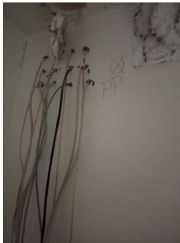
Figure 35: Penetration of the wall between the hallway and the garbage room, Image Credit: TDA
