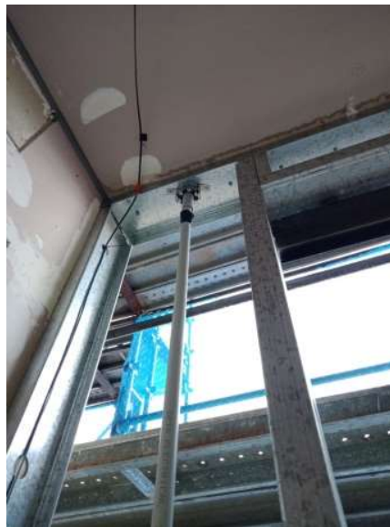
Figure 17: 25 and 32 mm conduit in a wall cavity with fire-rated collar, Image Credit: TDA
