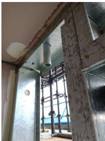
Figure 12: 32 mm conduit penetrating the floor, Image Credit: TDA
