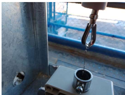
Figure 16: Connection of the stainless steel wire to fishing hook tracer, Image Credit: TDA
