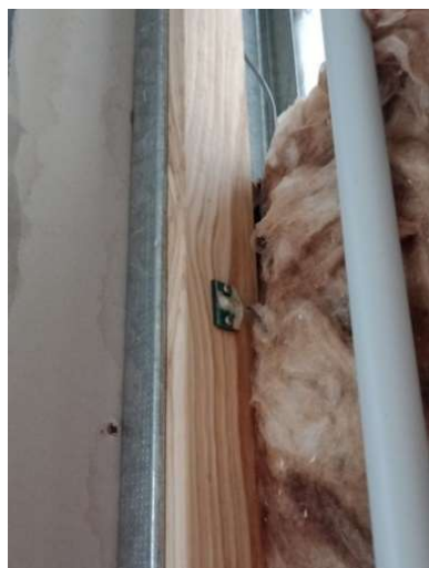
Figure 21: Radiata Pine stud with PMM sensor, Image Credit: TDA
