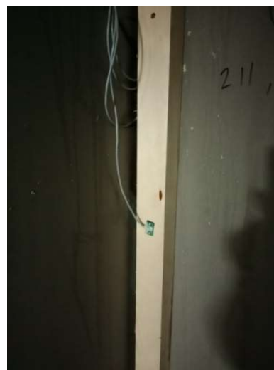
Figure 22: Spruce stud with PMM sensor, Image Credit: TDA
