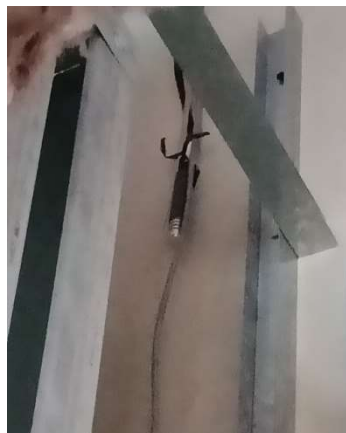
Figure 26: Relative Humidity and Temperature sensor behind a bathroom pod, Image Credit: TDA
