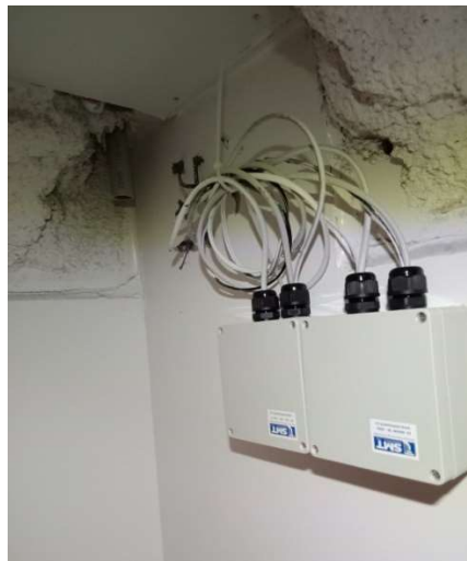
Figure 24: PMM wires penetrating wall in the garbage room and connected to A3 Data Acquisition Units, Image Credit, TDA
