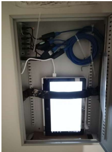
Figure 30: Locked box with the BIG installed, Image Credit: TDA
