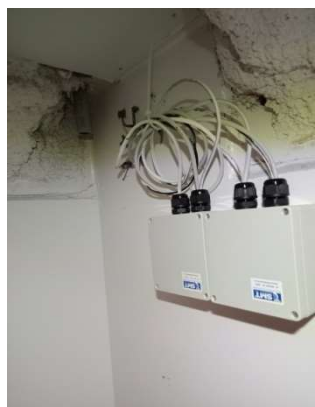
Figure 29: A3 Resistance unit in the garbage room, Image Credit: TDA
