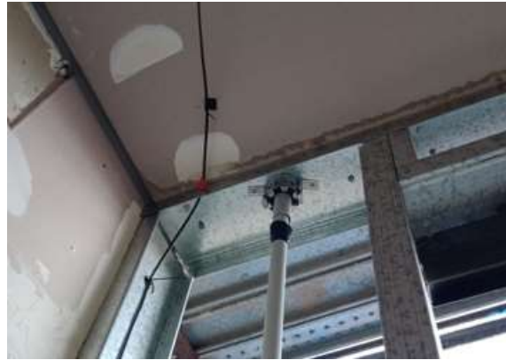
Figure 13: Fire Rated collar around the conduit, Image Credit: TDA
